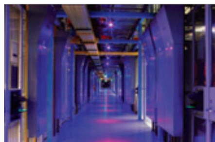
Colocation Space, Equinix SV2 Silicon Valley IBX® Data Center
